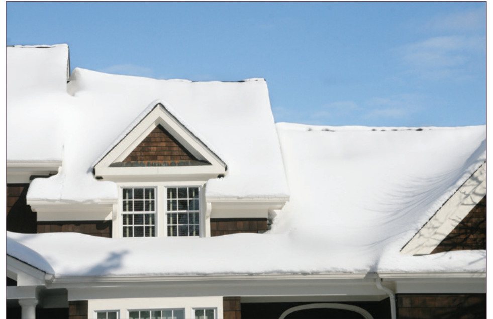
SNOW ON a roof may look idyllic, but too much weight can cause structural damage.
